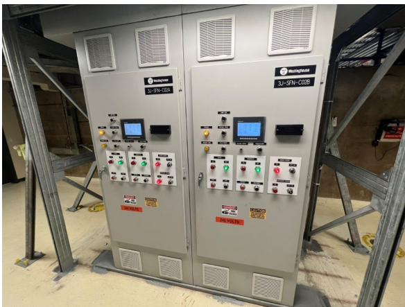
Next Generation MG Control Power Cabinets Installed
