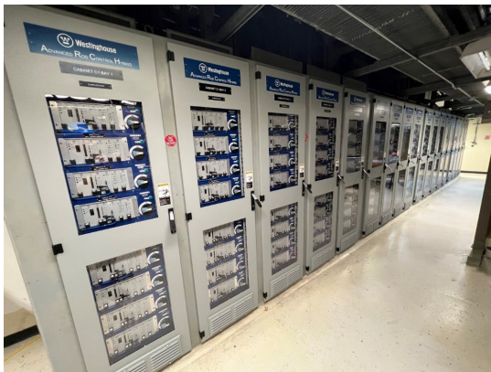
Advanced Rod Control Hybrid (ARCH) Cabinets Installed
