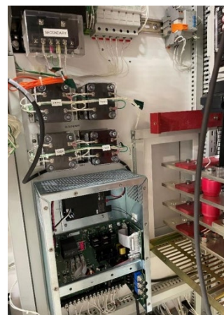
Typical Cabinet Internals with safety shields removed
